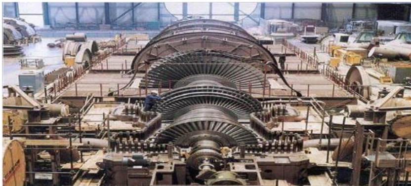
Figure: Steam Turbines
